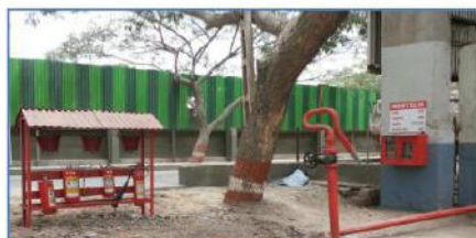
Proper Fire Hydrant System
